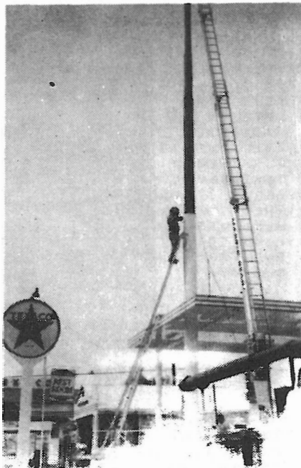
FIRST WELD ON TELESCOPIC STANDARD FOR HUGE TEXACO SIGN 55 FEET OVER NEW BOB WILSON STATION. HE HAS TWO MORE TO MAKE. THEN GOES TO SECOND STANDARD FARTHER BACK. FOR SAME OPERATION. RAISING OF SIGN IS BIGGEST TASK. BOB'S NEW STATION, NEARING COMPLETION, IS A FINE ADDITION TO BUSINESS AREA.
